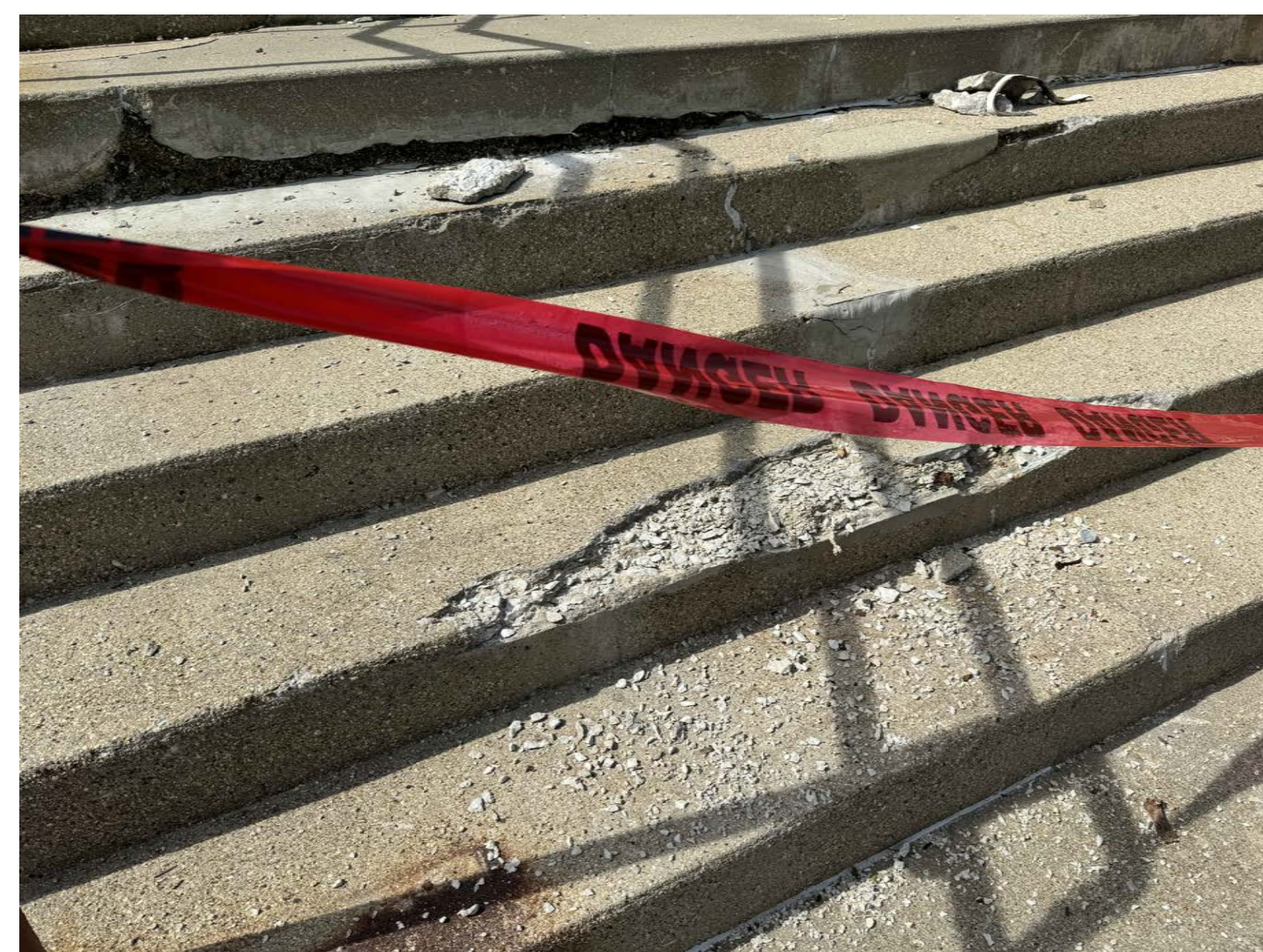
FRONTAL VIEW OF STAIRS - ZOOM IN ON SPALLING
